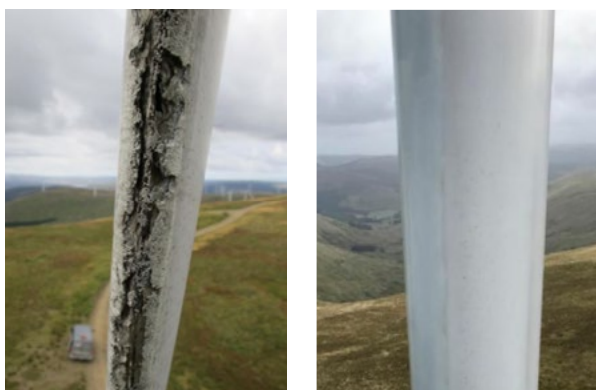
Blade damage, before and after repair.
