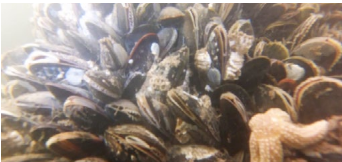
BIO-FOULING OF TURBINE TOWER
